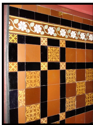
Figure 7 – Whetstone tiles at Leeds Grand Theatre. 9
