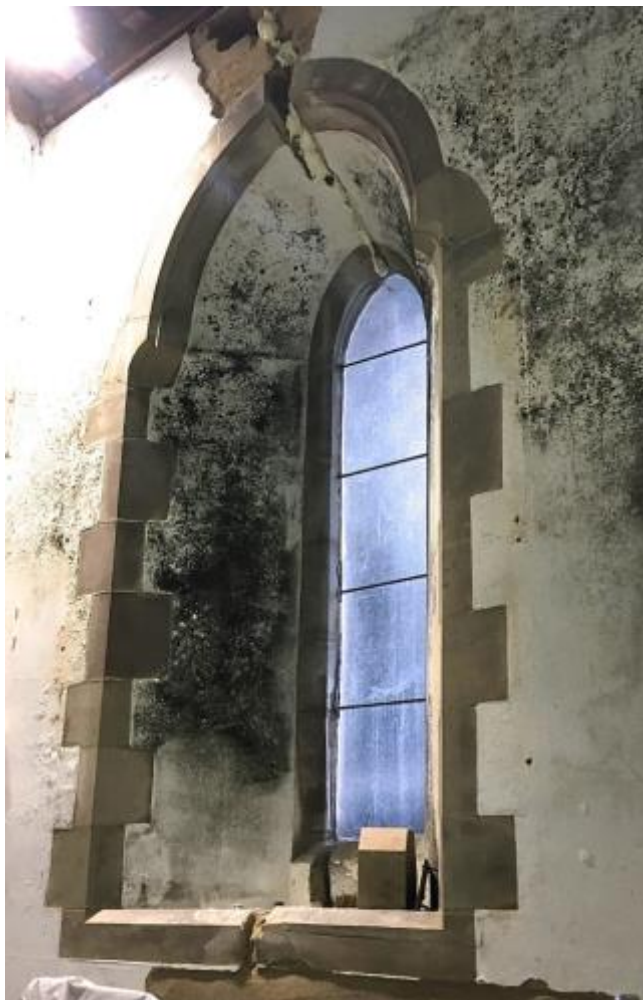
The Hope window frame during repair, the crack and mould are visible and the new sandstone block is waiting on the sill.
