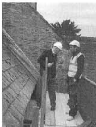
On the scaffolding beside the chancel roof and an area of removed tiles.
