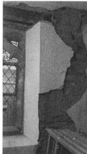
The vestry has been cracking severely with the subsidence too. The corroded metal window lintels also need replacing.
