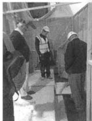
In the chancel, checking out the new steps and floor under construction for the ramp.
