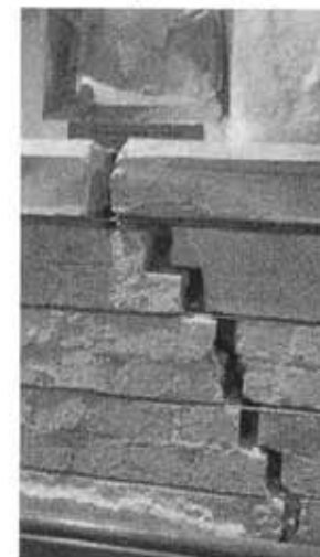
The worst crack in the chancel, going across the Hope window frame; during the visit the daylight could be seen through this crack! The metal wires are reinforcements in the repair.
