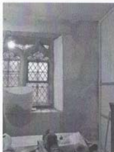
Plastering over the vestry crack repairs and replaced lintel above the window.
