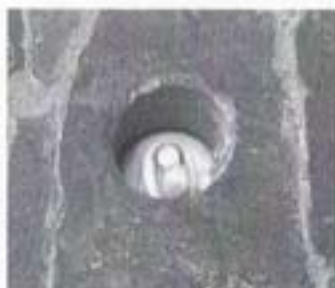
The end of one of the metal supporting rods in the chancel walls before it was sealed.
