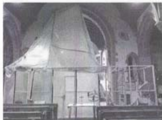
The 'canopy' put up to protect the body of the church from dust and dirt coming down at the end of the works.
